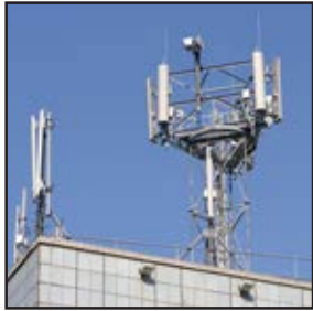
Communication Tower Security
